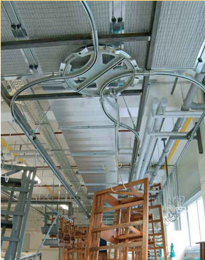
Overhead conveyor system with Müsing spider assembly.
